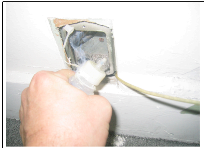
Identification of air leakage pathway in an electrical outlet box with chemical smoke.
