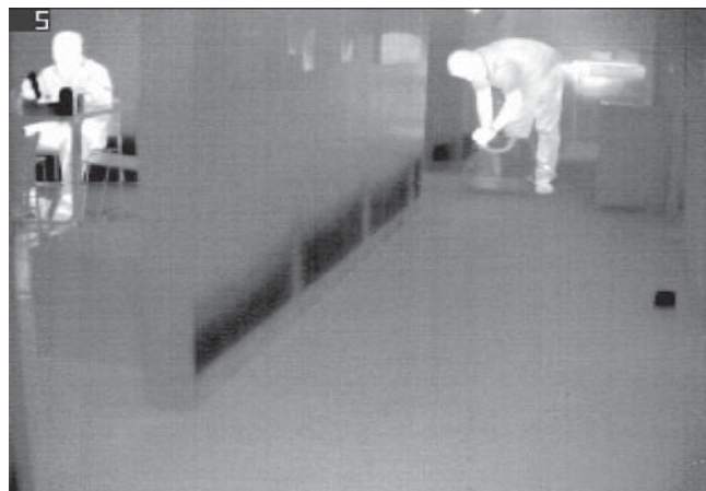
Fig. 3.14 The importance of a gap at the base of a gypsum board wall
