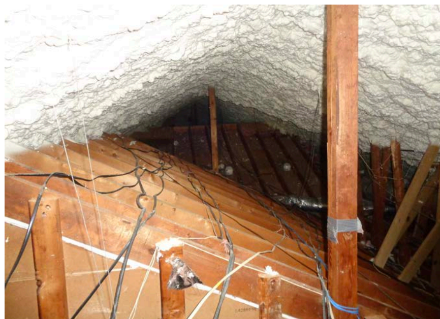
Figure 1. Photograph of the SPF applied to the underside of the roof deck in the Attic of home GA-2.
